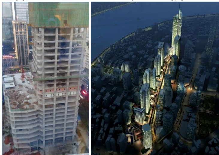
Photographs of actual ICC construction site and artist impression of Chongqing Financial Street
