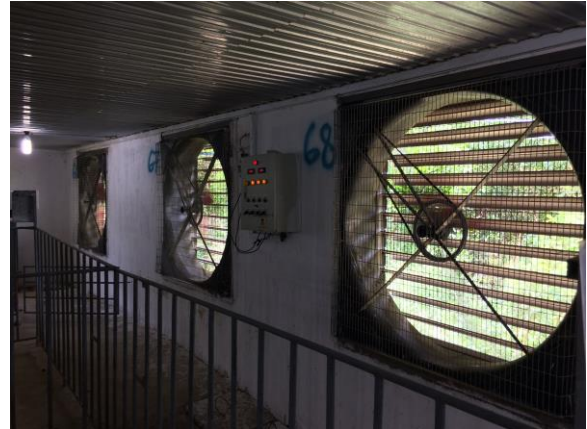
Figure 4. Fans to regulate air temperature
